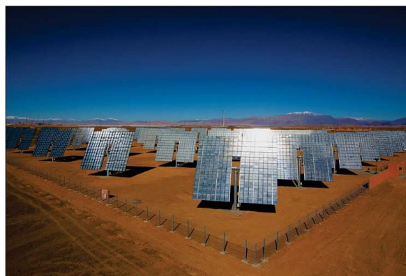
Fig. 8. CPV plant in Noor IV Ouarzazate
