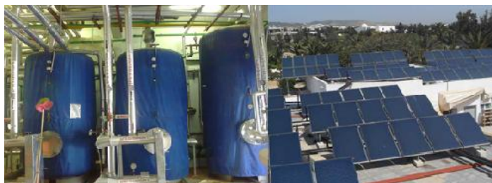
Figure 1. The studied solar installation.
